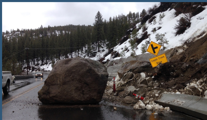
Extreme weather increases the risk of landslides damaging roads. Photo: Nevada Department of Transportation
